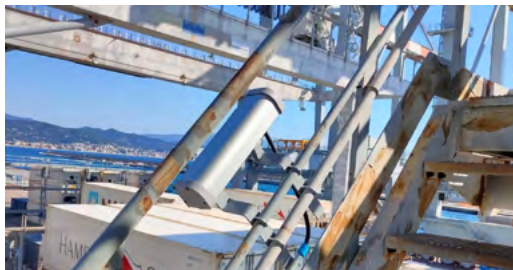
(Picture of a Progress light installed)
